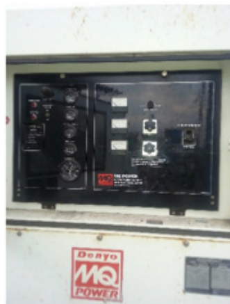
GENERATOR CONTROL PANEL
