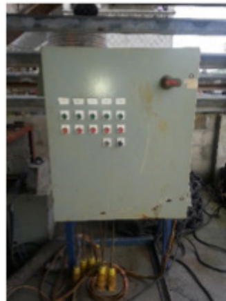
PLANT CONTROL PANEL
